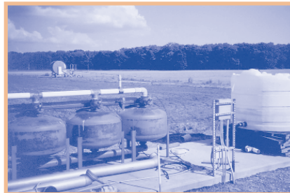
Irrigation pumps with filters used for spraying irrigation.
